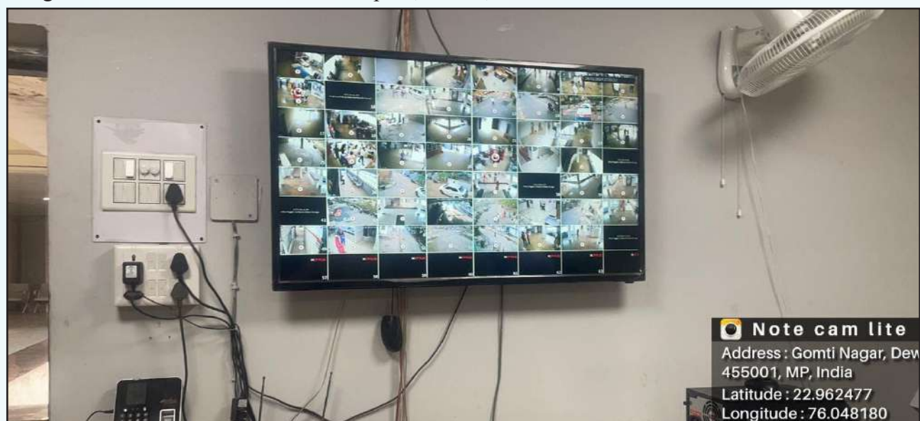
Image 16: CCTV control room at MG hospital, Dewas, M.P.
